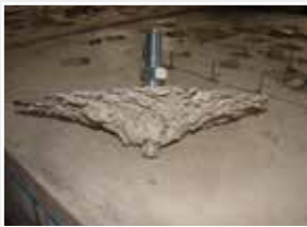
CONCRETE CONE FAILURE
